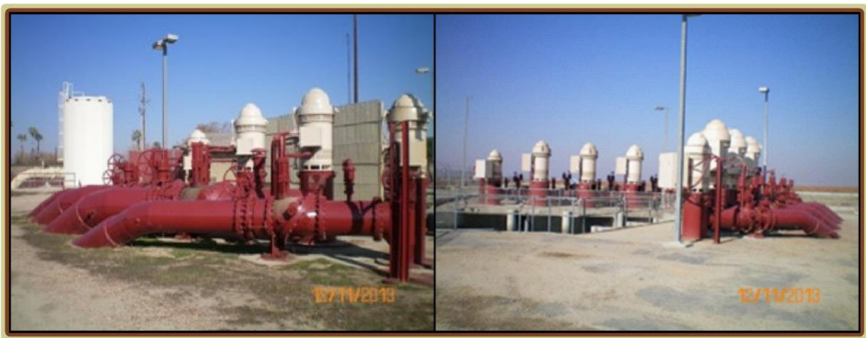
Figure 3A and 3B. District Pump Station "A" and "B"
