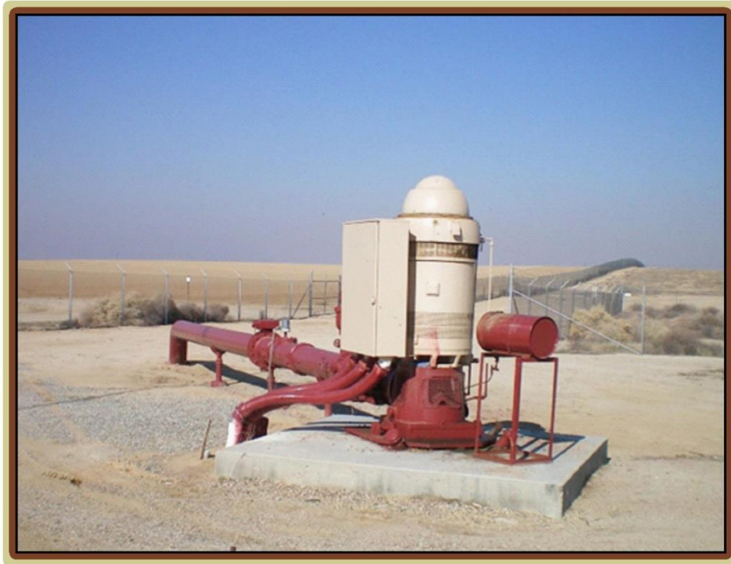
Figure 10. Typical Cawelo District-Owned Groundwater Well
